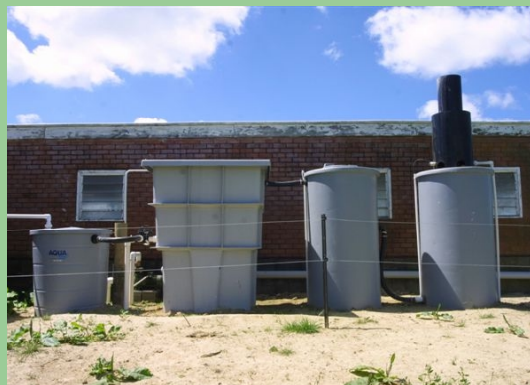
IRON & MANGANESE SYSTEM FOR BORE WATER
