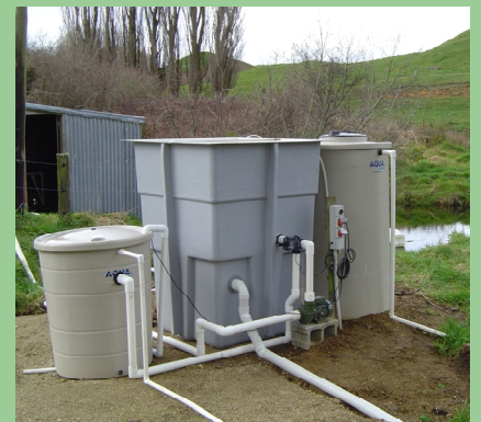
TURBIDITY REDUCTION SYSTEM FOR POND/DAM WATER
